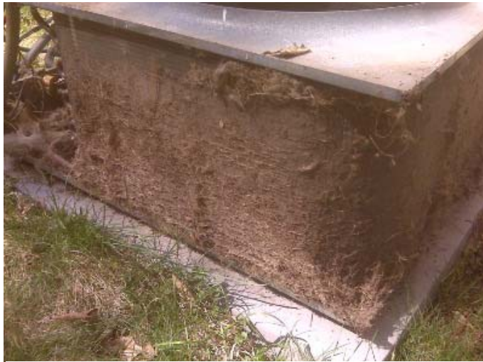
Figure 3. Condenser Coil Fouling
