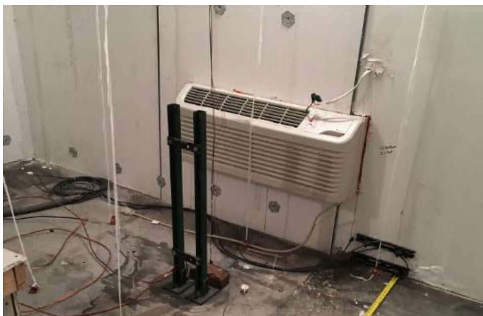
Figure 89 - Camera view of PTAC mounted in the center of the wall
