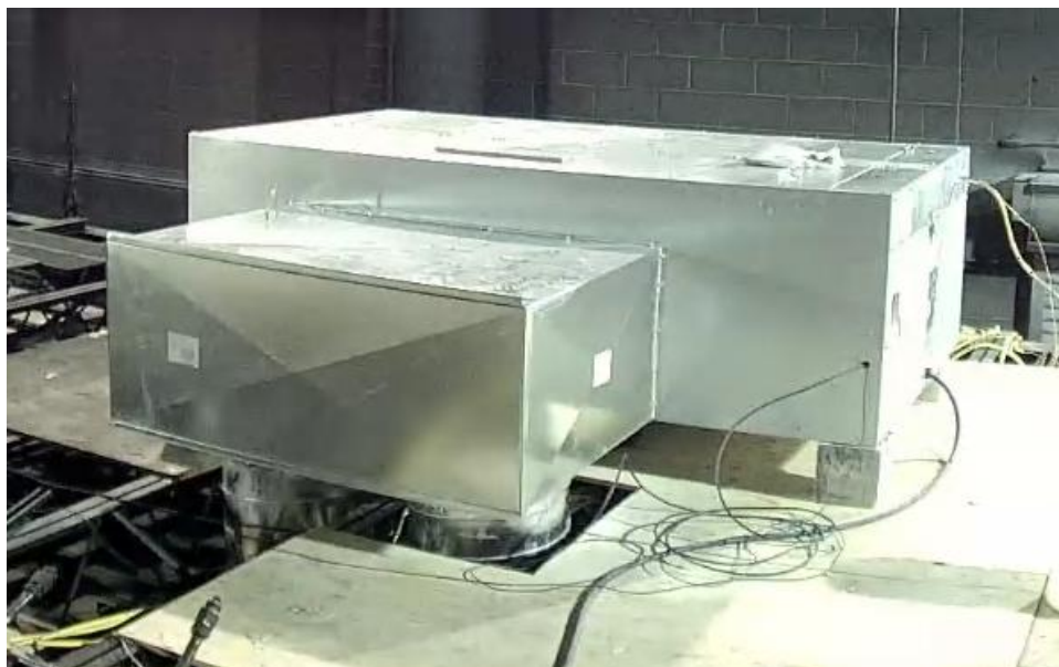
Figure 114 – Roof top unit (supply side)
