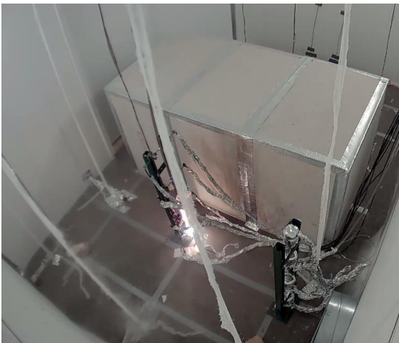
Electric arcs after release: 4:02
