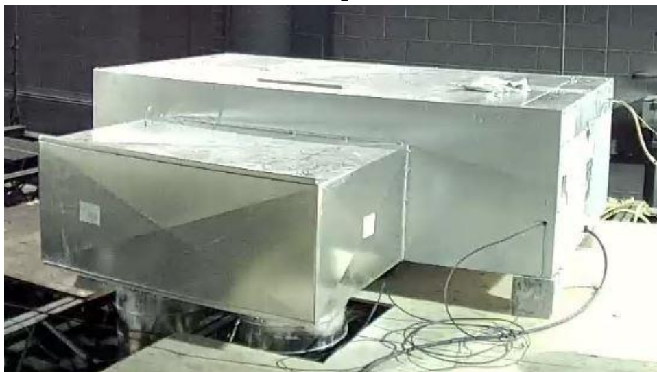
Figure 167 – Rooftop Kitchen Unit
