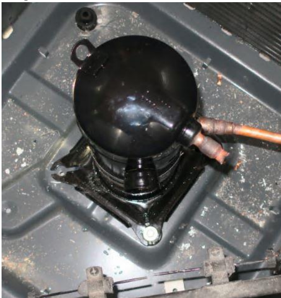
Figure 171 – Outdoor Compressor (Hermetic Electrical Pass-Through Terminal Failure Tests)
