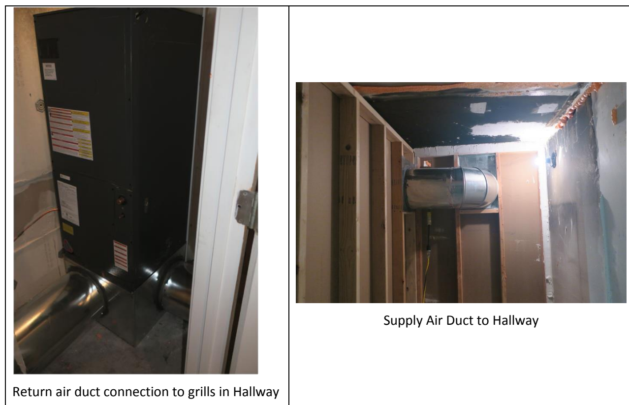
Figure 136 – Return Air and Supply Ducts Air connecting to Air Conditioning Unit
