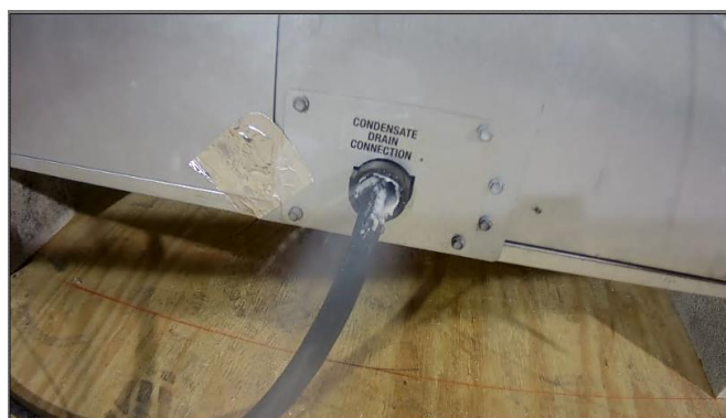
Condensate Drain on RTU
