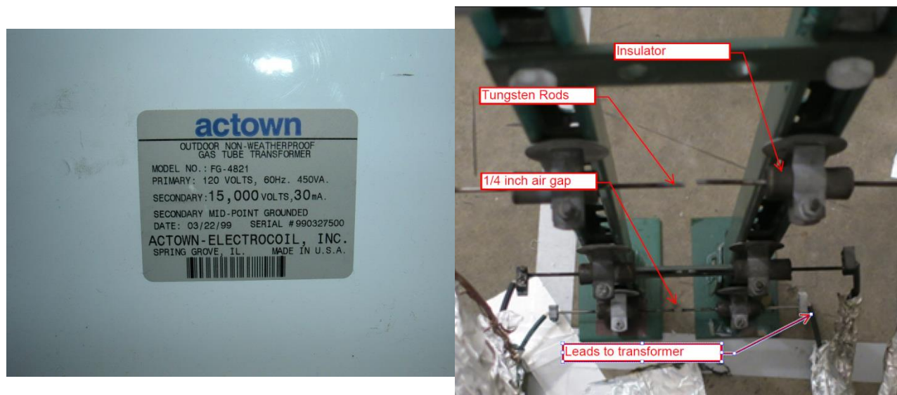
Figure 14 – Gas tube transformer and arc gap
