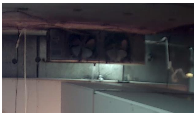
It appears that liquid refrigerant is dripping from the drain at 63 seconds after the start of the discharge.
