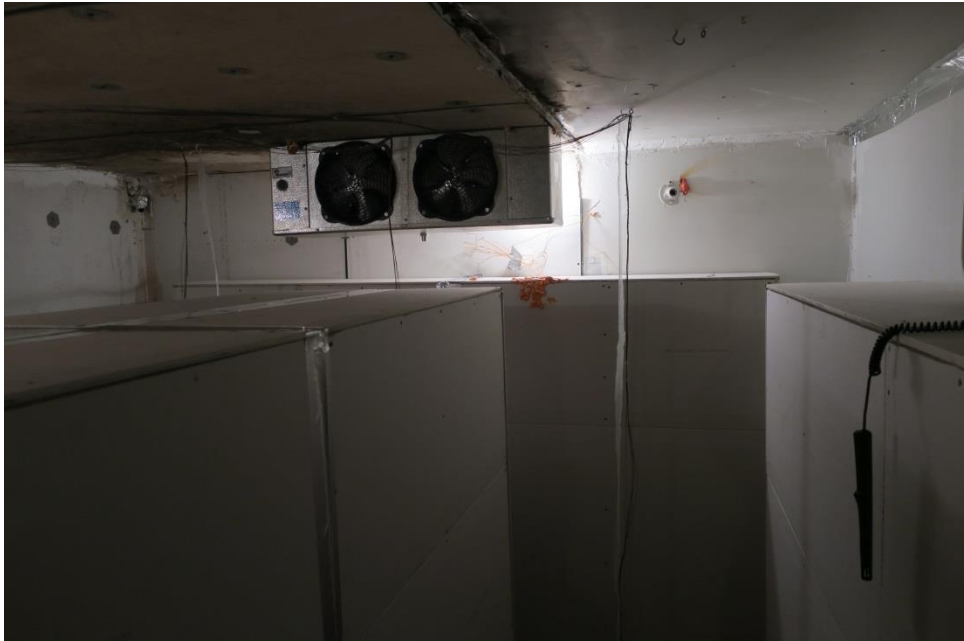
Figure 126 - Camera view of evaporator mounting and obstructions
