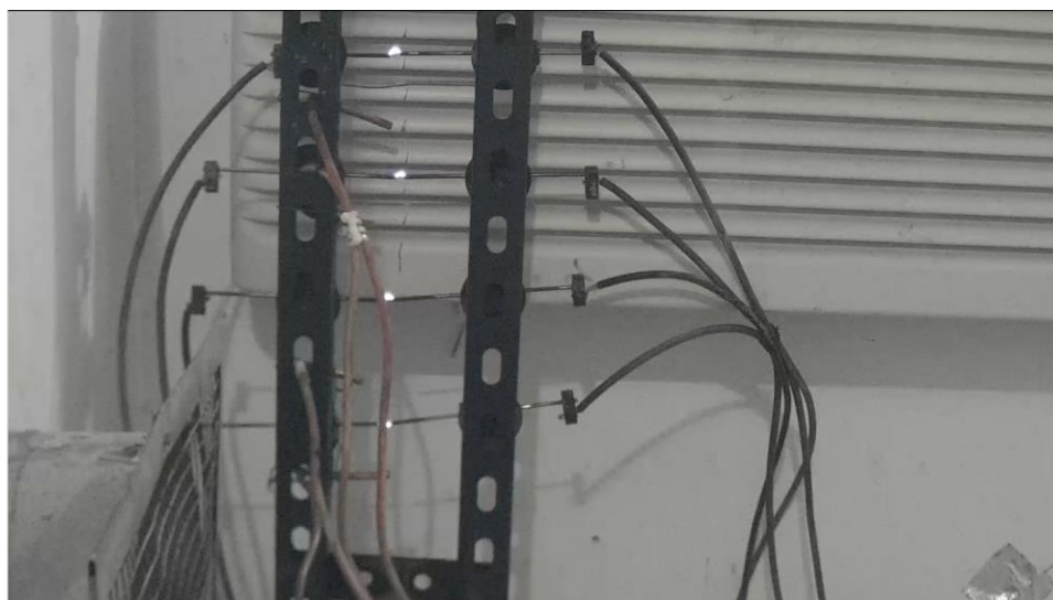
Figure 103 – Electric arcs and refrigerant sampling tubes immediately in front of discharge location
