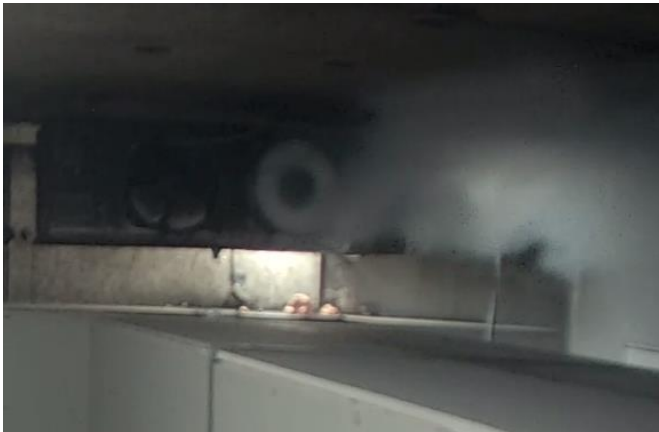
The discharge in the coil face caused the fan to rotate. Note the frost buildup on the right-hand fan blades.
