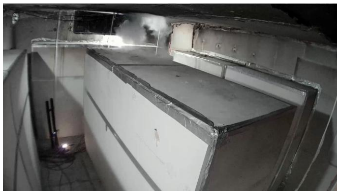
Ceiling camera view of the discharge showing the condensation cloud at the ceiling level.
